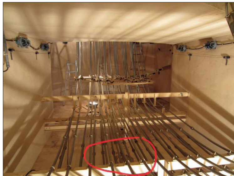
Figure 5: RPV cavity floor drain opening protected with sieve (marked)
