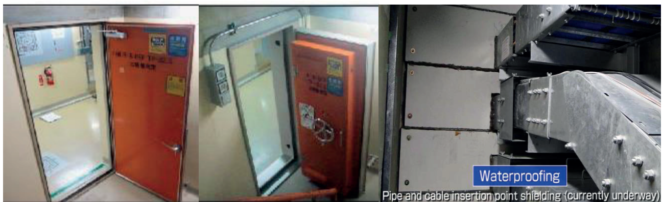
Figure 4 Example of measures to prevent flooding of the critical equipment room and water tight cable conduits penetrations: Kashiwazaki-Kariwa NPS. (Source: TEPCO www.tepco.co.jp/en/nu/kk-np/safety/flood-e.html , tepco.webcdn.stream.ne.jp/.../201404-e.wmv )
