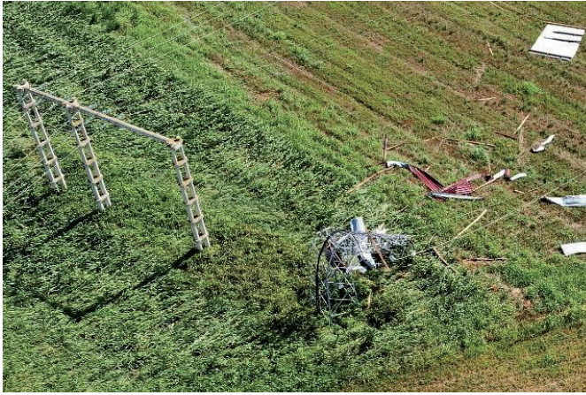
Fig.13. Damage of 110 kV OHL near substation
