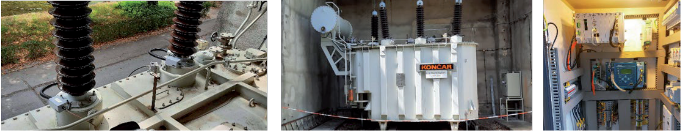
Fig. 6. Transformer Monitoring Installation
