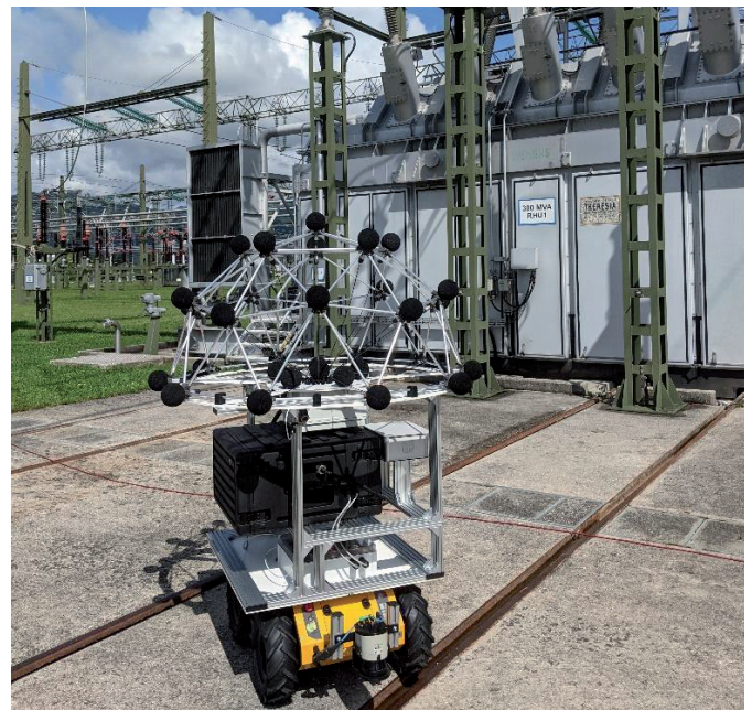
Fig. 8: Microphone array mounted on a mobile robot during measurements in a substation.
