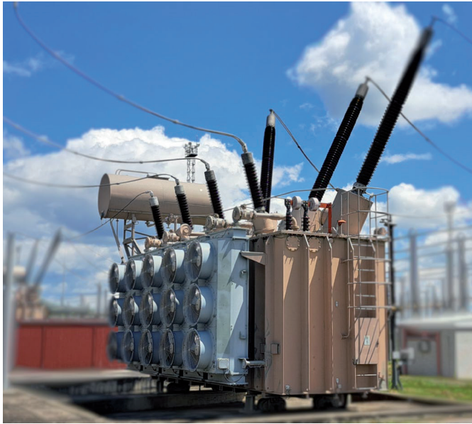
Fig. 1. Image of the transformer from which the data was collected
