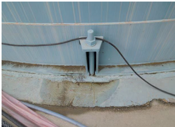
Fig. 2: Possible signs of leakage on tank 1
