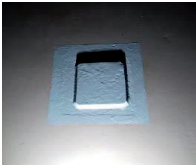
Fig. 13. Coated steel plate inside CY tank
