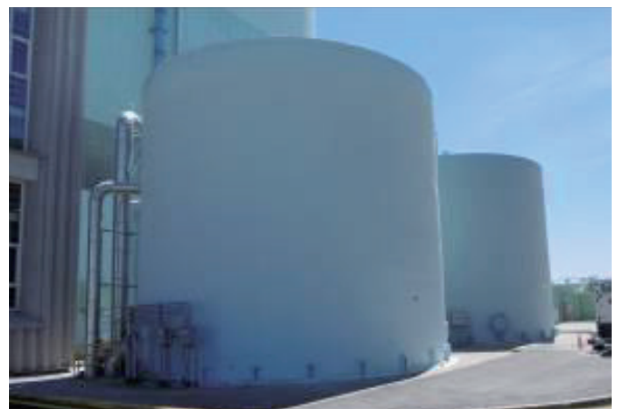
Fig. 1. Condensate storage tanks 1 and 2
