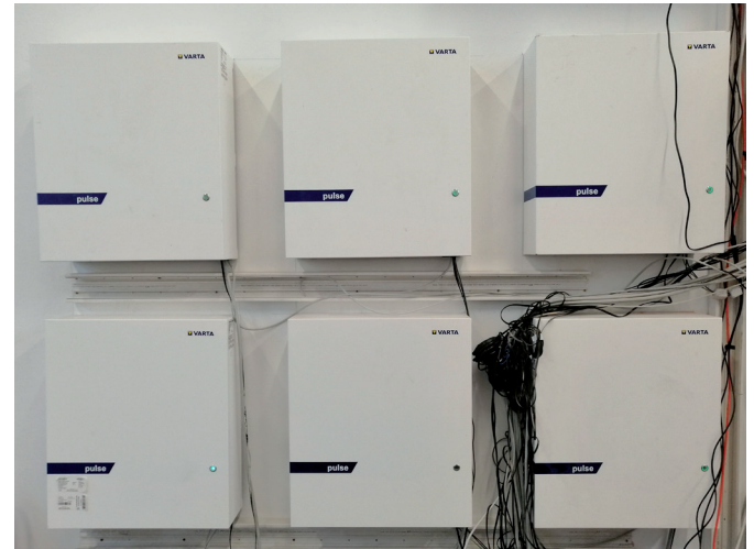
Fig. 2. VARTA Pulse 6 battery units in SGLab
