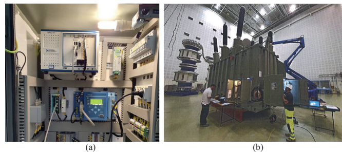
Figure 3: TMS+ system (a) installed in a 100 MVar 220 kV VSR (b).
