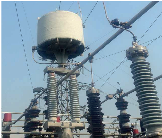
Figure 12. (a) Isometric view of the rigid tubular buswork system, (b) Tubular rigid conductor installed between two disconnectors and going in-between two post insulators for line trap installation
