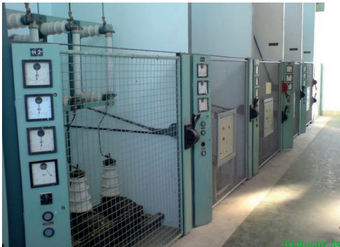
Image 2 10 kV plant and protective cabinets for installations before reconstruction
