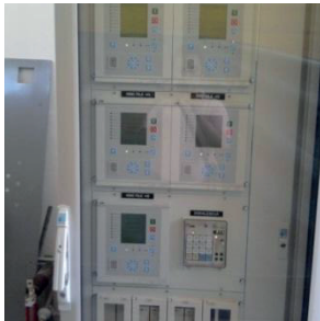
Image 10 Protection cabinet of the 35 kV plant
