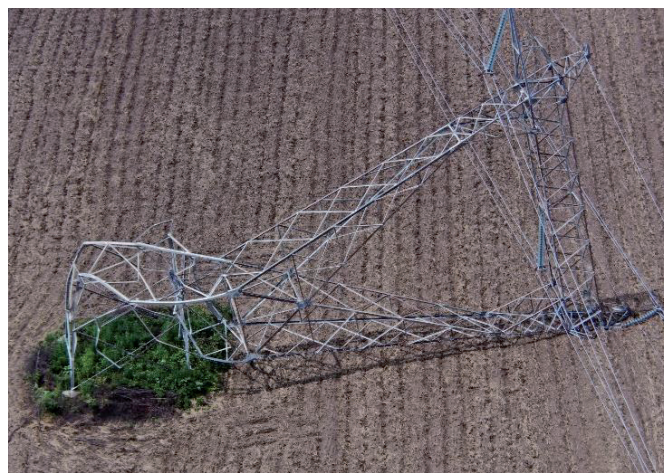
Fig. 12. Damage on OHL 400 kV Ernestinovo – Sremska Mitrovica located in transmission area OS (tower no. 120) due to storm on July, 2023
