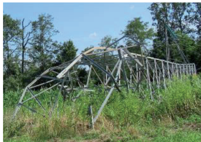
Fig. 11. Damages on OHL 220 kV Međurić – TPP Sisak located in transmission area ZG (tower no. 99) due to storm on July, 2023
