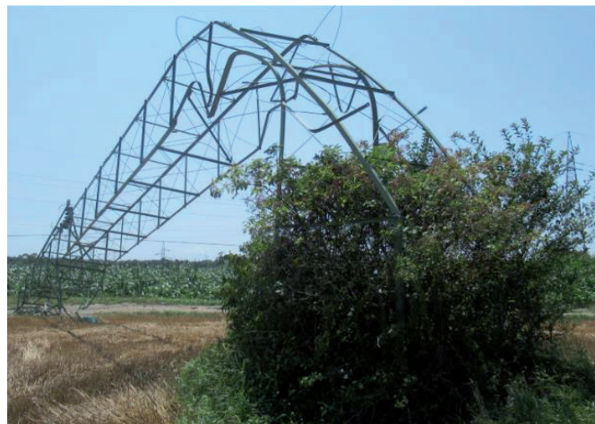
Fig. 10. Damages on OHL 110 kV Međurić – Daruvar located in transmission area ZG (tower no. 3) due to storm on July, 2023
