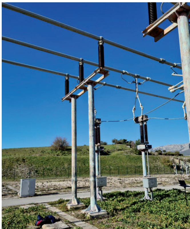
Fig. 10. A view to a part of 110 kV bus
