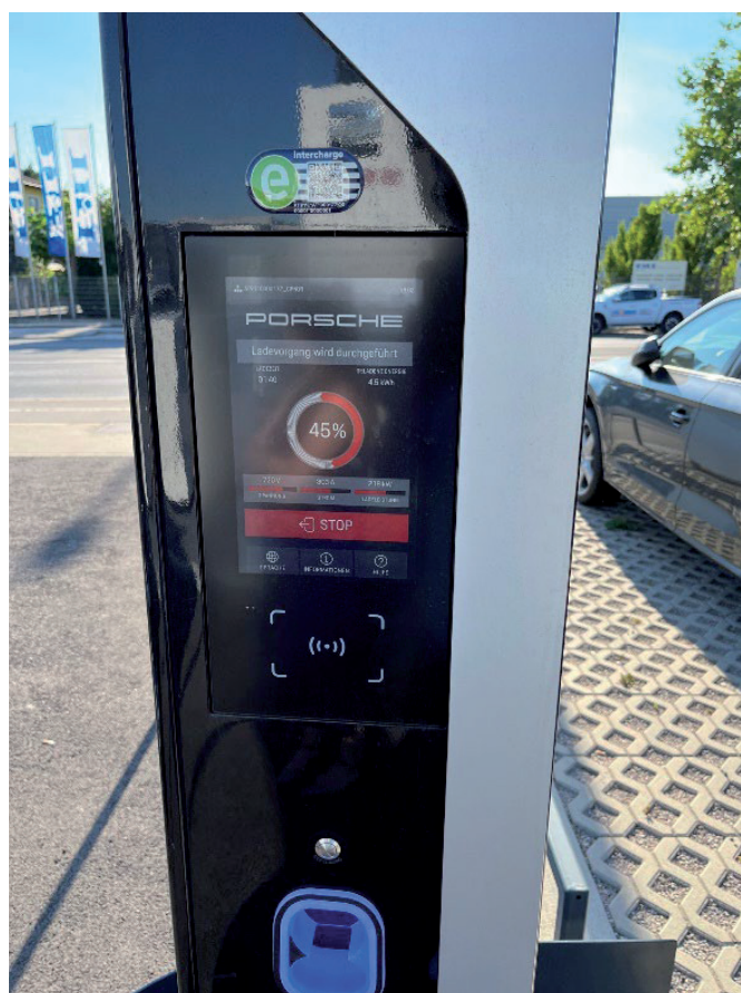
Fig. 1 Porsche Zentrum Wien-Liesing charging station
