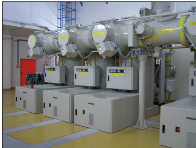
Fig. 2 View on one of the GIS 110 kV substation Dobri in which EMC conditions have been investigated
