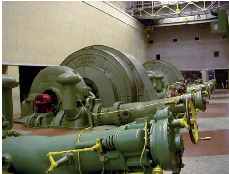
Figure 1 - Hydro-generators (35 MVA) with Pelton turbines
