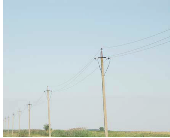
Fig. 5. 6 kV overhead line in Kuban utility (Russia) equipped with LFA-Ms.
