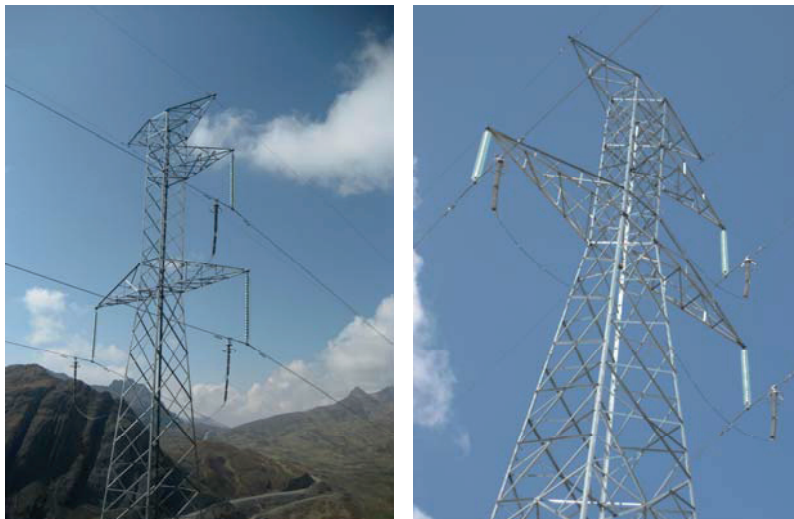
Figure 3 – Class 2 TLA with rated voltage of 192 kV installed along 220 kV line
