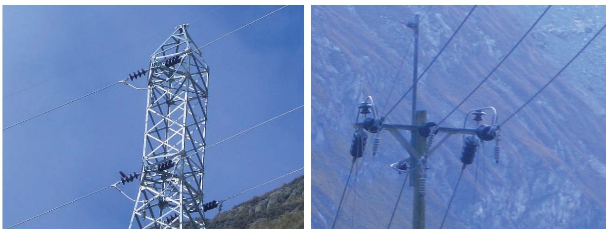
Figure 2 – Class 2 arresters installed on 23 kV overhead shielded distribution network
