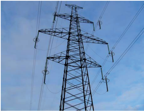
Figure 5. “Trouble tower” with arresters installed in both circuits and in all 6 phases.
