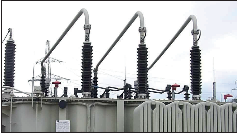
Figure 5: Tubular connections between the switchyard and 123 kV bushings
