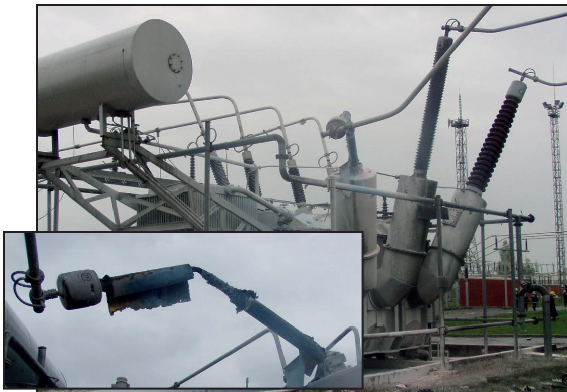
Figure 9: Bushing terminal failure in 2003 and traces of fire on the 300 MVA, 400 kV autotransformer; The right-hand bushing in the figure was replaced after an incipient failure in 1994. Detail shows the bushing debris and the tubular connection dilatation compensator
