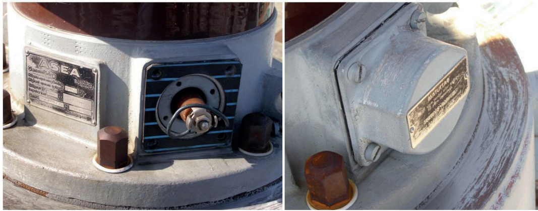
Figure 17 – Measuring tap on ASEA bushing from 1965.
