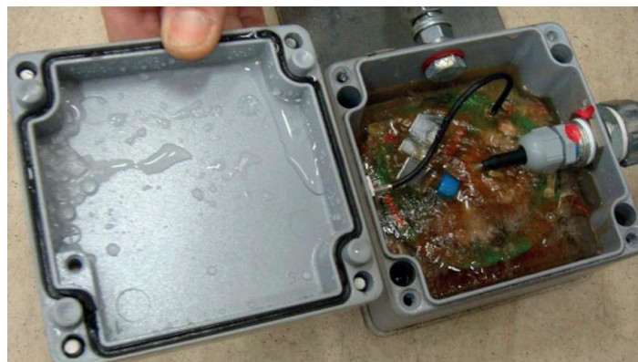
Figure 12 – Problem of water penetration
