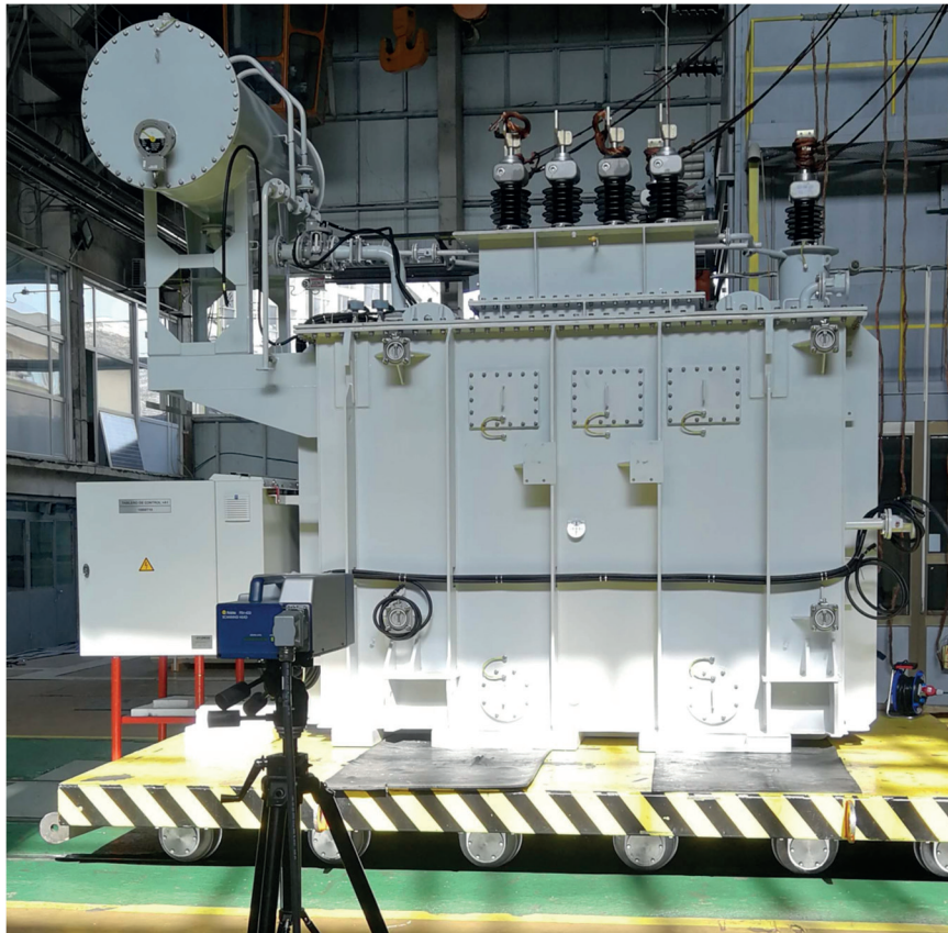
Figure 3 Measurement of the vibration of the transformer tank
