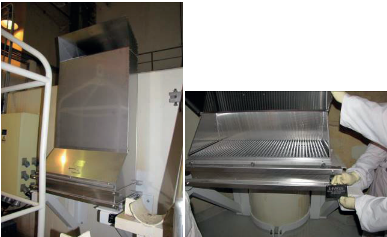
Figure 1: An example of the installed PAR unit in NPP Krško
