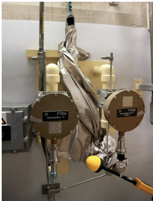
Figure 2 Retesting of the Pressure Transmitters with Provisionary Shielded Flexible Conduit
