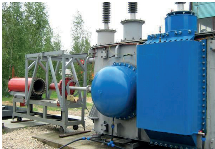
Figure 7 – Autotransformer with DPS before tests
