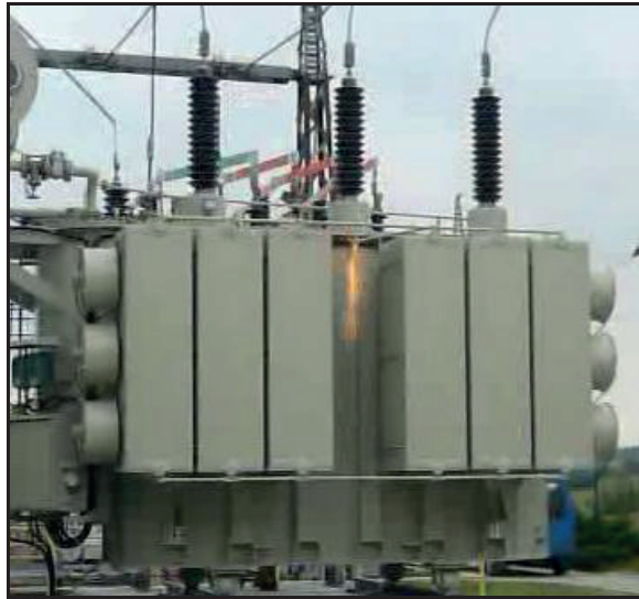
Figure 2: Sparks on tank during inrush current, transformer 40 MVA, 110 kV
