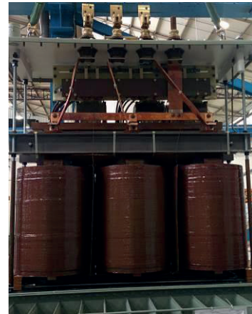
Figure 5 – RDT after short circuit test
