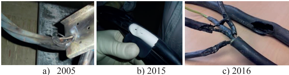
Figure 12: Failures due of LV power cables found with IR test
